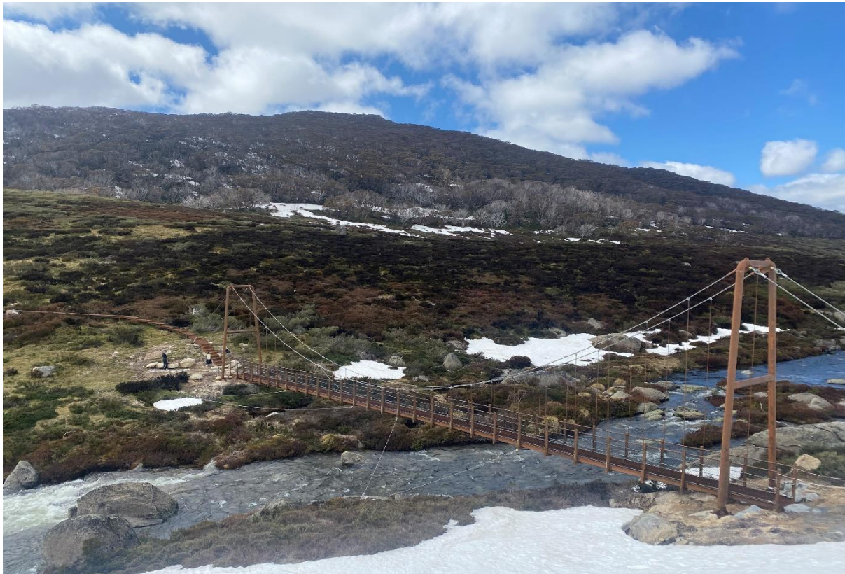
The new bridge over Spencers Creek in the Guthega-Charlotte Pass section of the new Snowies Alpine Walk.
