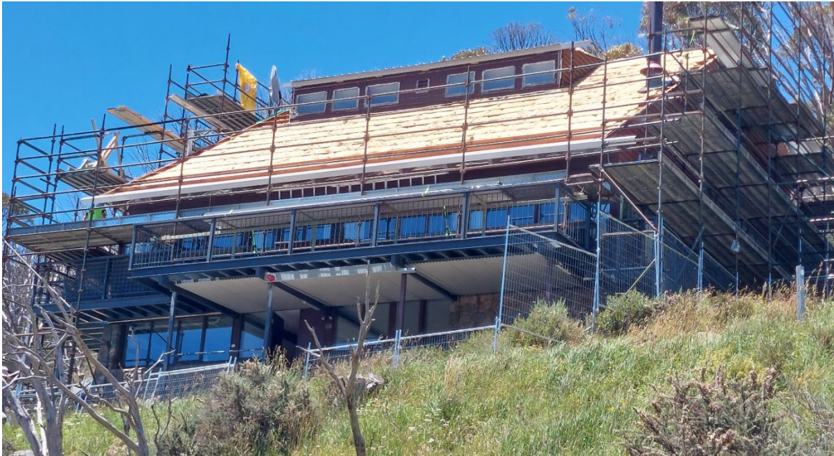
Our lodge was wrapped in scaffolding in January. The first task was to replace the roof.
