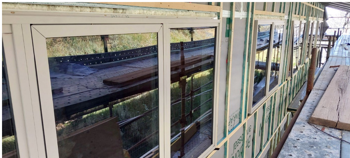
Top: New insulation is installed in the rear wall. Bottom: Bedroom windows are installed and the wall is ready for cladding.
